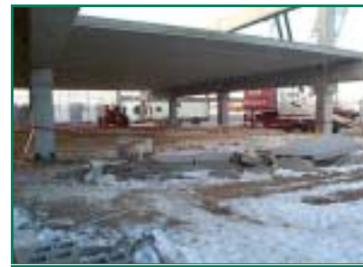
Geotechnical exploration, construction testing and special inspections are part of Pinnacle's Construction Management Services.
