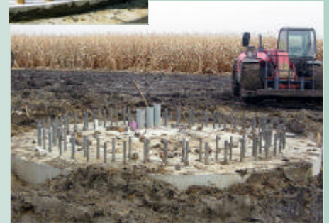
Concrete pads serve as the structural base for wind turbine towers.
